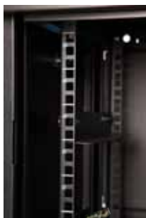
Earthing Studs/Cable Locations Provided
